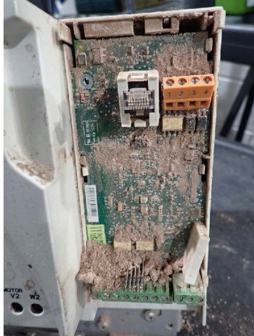
▲ ABB Variable frequency drive (VFD) drive before decontamination
