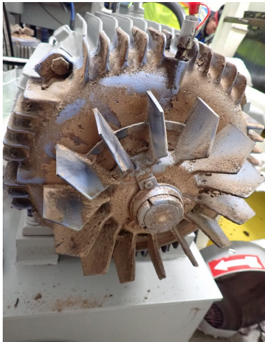
▲ Motor before decontamination
