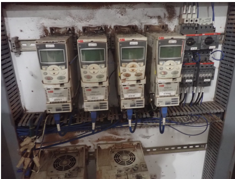
▲ SCHOLD mixer control cabinet before decontamination
