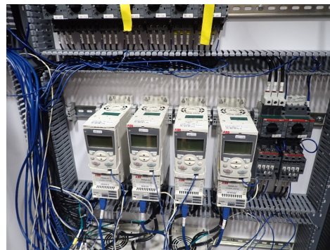
▲ SCHOLD mixer control cabinet after decontamination
